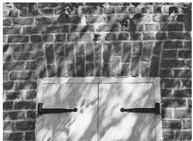
FIGURE 31. Flat arches typical of windows on south, east, and west elevations of main block of house.
