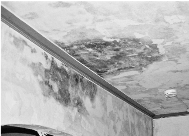
FIGURE 55. Water-damaged ceiling in Room 102.
