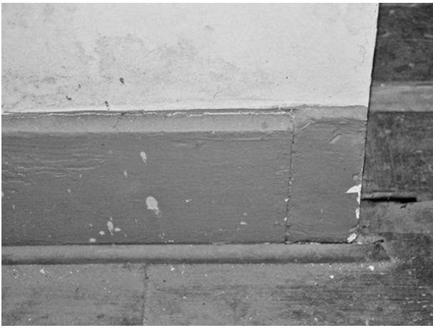
FIGURE 53. Baseboard on north wall of Room 102. Note that right end is plaster.
