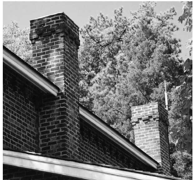
FIGURE 35. Chimneys on north elevation of second story. Note that the left chimney has a galvanized metal cap.
