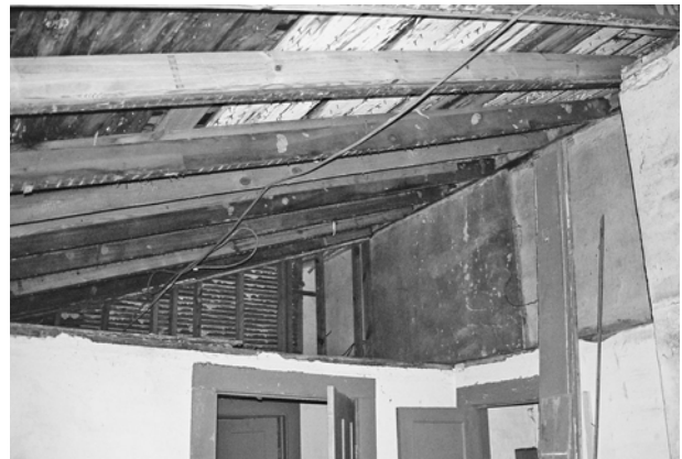
FIGURE 62. View of upper portion of east and south walls in Room 105 and exposed roof framing above.
