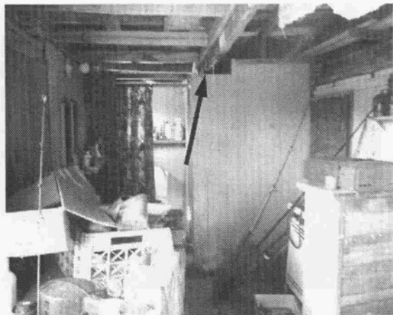
Figure 42 View northwest in Room 105. Arrow marks header at outside of historic porch. (NPS-SERO-CR, 2002)
