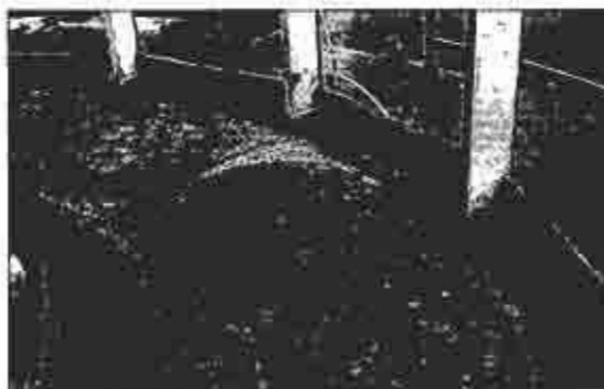
Figure 10 1989 USCOE photo showing missing lantern deck prisms.
