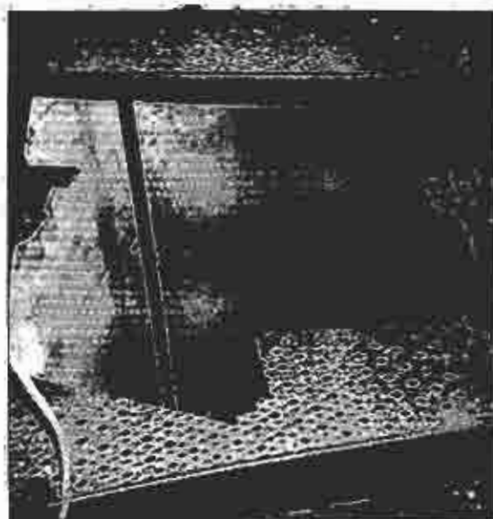
Figure 12 USCG close-up photograph of damage to stair treads, 1992.
