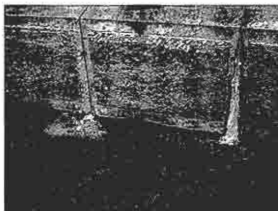
Figure 44 Detail of foundation showing mortar leaching.
