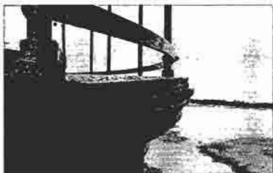
Figure 9 1989 USCOE photo showing deterioration of exterior edge of lantern gallery.
