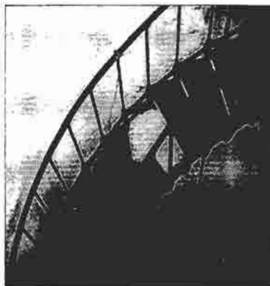
Figure 13 USCG photograph of damage to stair treads, 1992.
