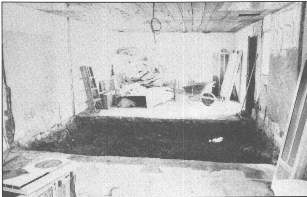
Figure 1.10 Interior of Building 15 after razing, showing removed central section of concrete floor.
