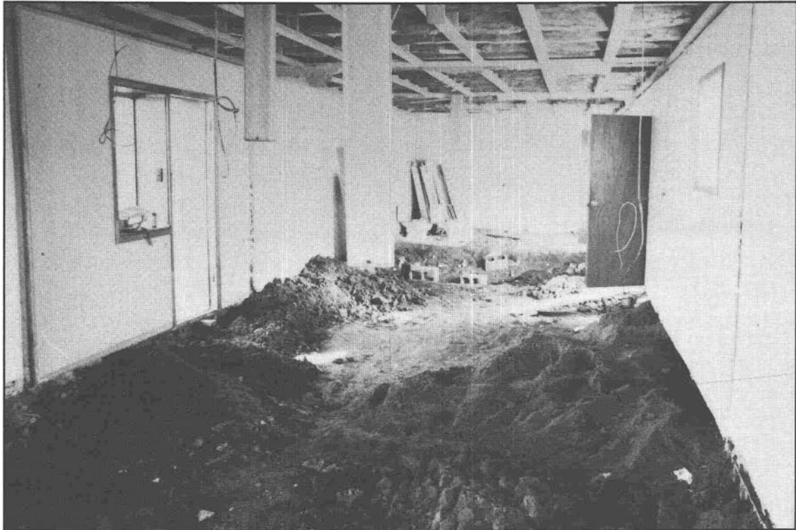
Figure 1.8 Interior of Building 14 after razing. Fill dirt is being added preparatory to pouring a concrete slab floor.
