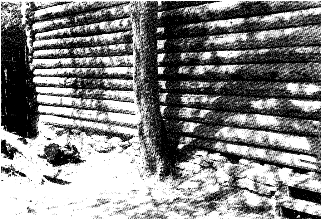
In 1986 stucco covered the east wall of the garage. A tree grew out from the stone foundation at the south end of the east wall.
