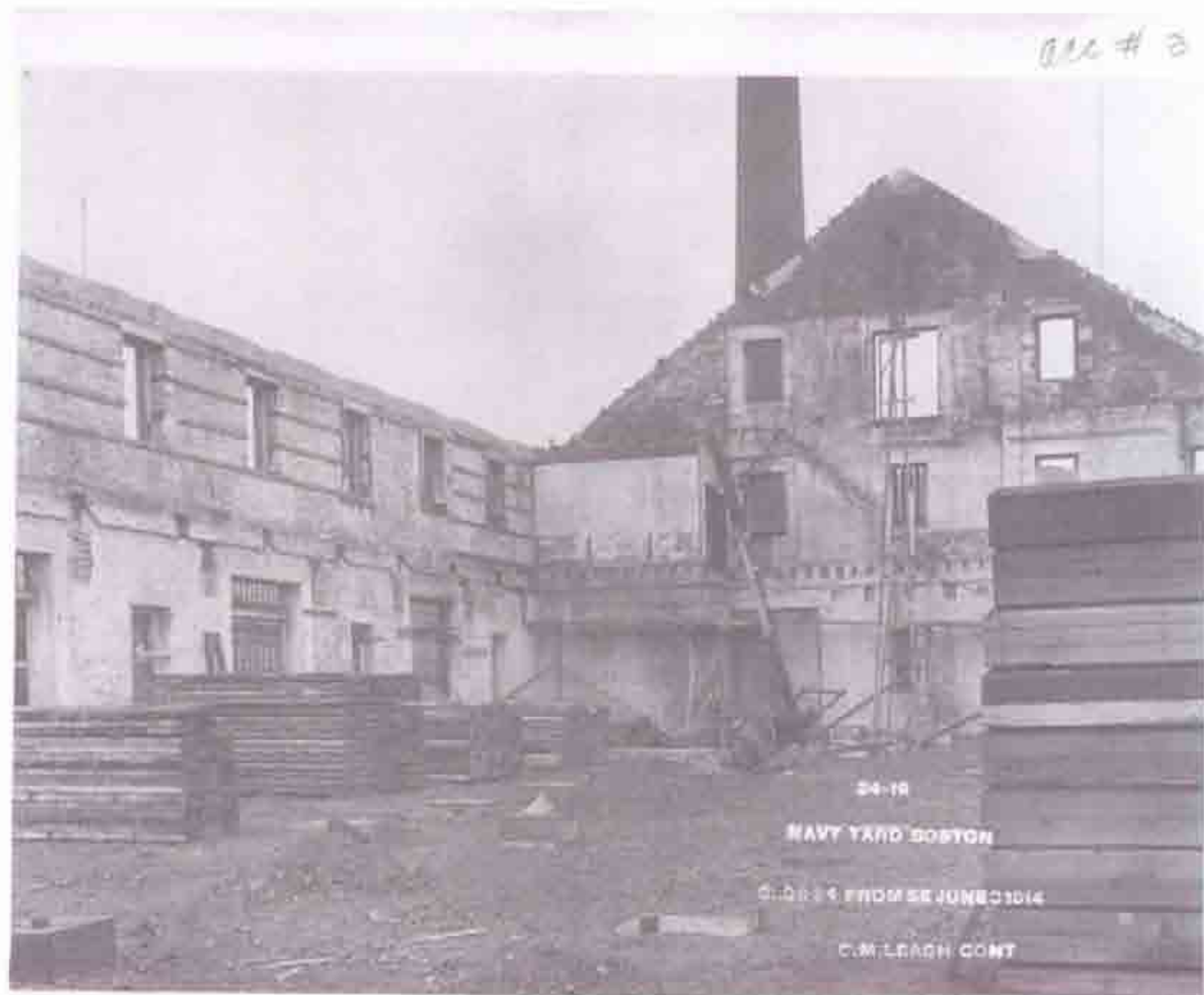
Fig. B-20 Photo "24-19 NAVY YARD BOSTON BLDG 24 FROM SE JUNE 8 1914 C. M. LEACH CONT". First floor interior, looking northwest. Materials stocked in building for reconstruction.
