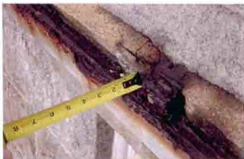
Fig. 32. West elevation cornice stone. Note rust jacking at Z channel.
