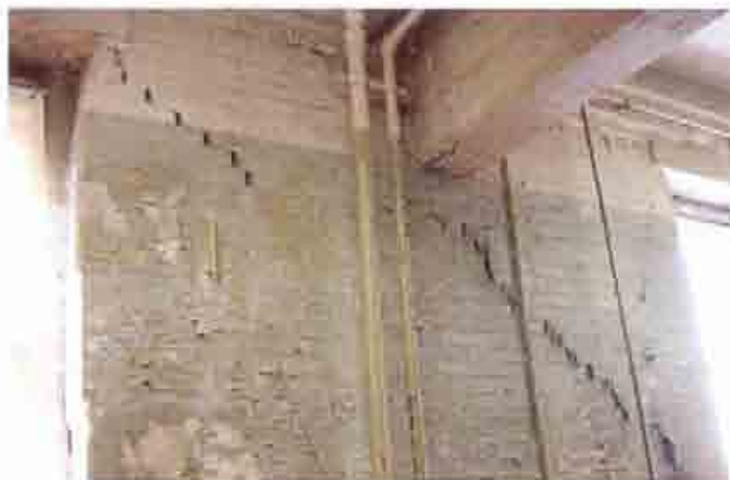
Fig. 29 Step crack at west exterior wall. Interior location of Fig. 20.
