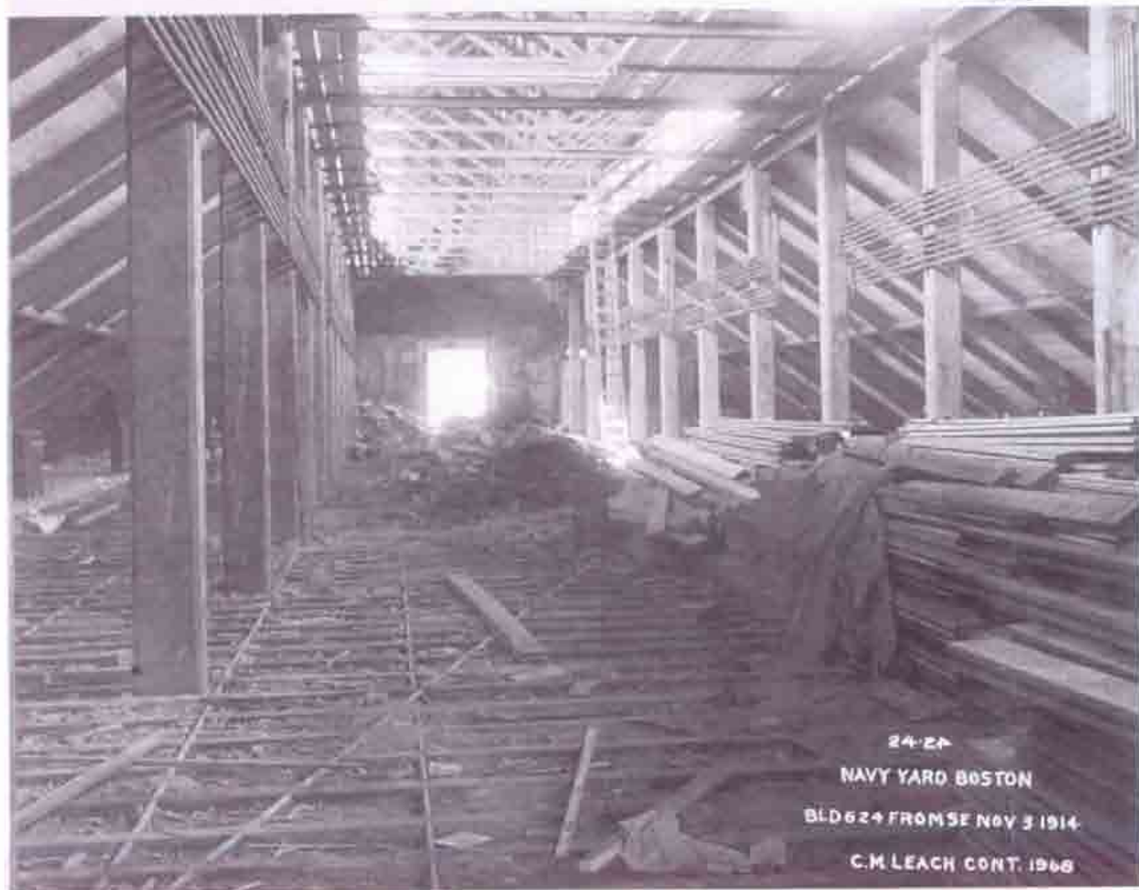
Fig. B-26 Photo "24-24 NAVY YARD BOSTON BLDG 24 FROM SE NOV 3 1914 C. M. LEACH CONT. 1968": Third floor interior, looking north. Heating pipes installed, concrete poured around columns, roof sheathing complete, materials stacked on floor.
