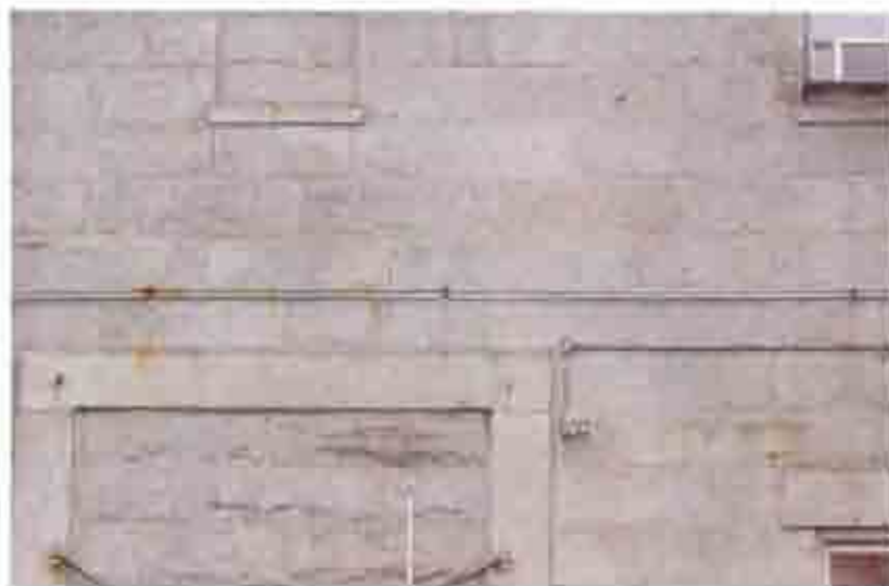
Fig. 10. Old fasteners for surface elements long since removed remain in the granite, leading to staining of the surrounding stone.
