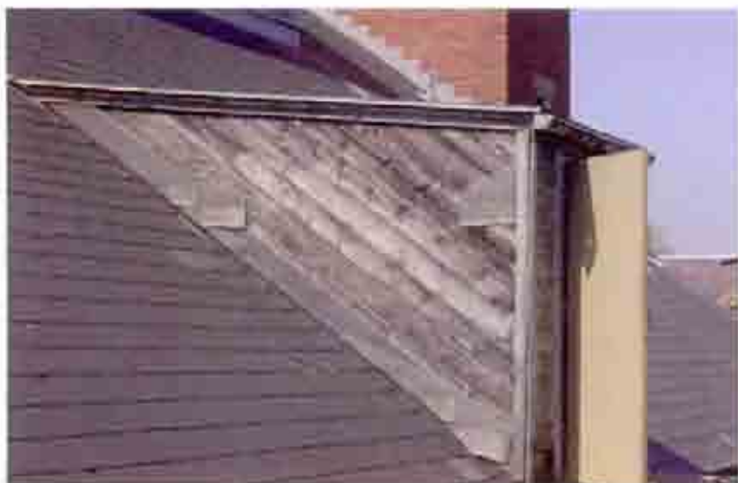
Fig. 15 The east elevation dormer is in fair condition.
