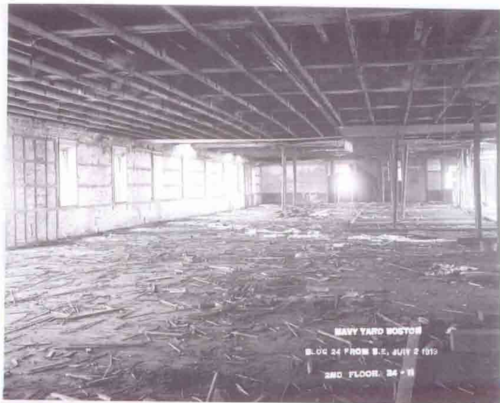
Fig. B-12 Photo "NAVY YARD BOSTON BLDG 24 FROM S.E. JULY 2 1913 2ND FLOOR 24-11". Interior photo of original wood floor system with temporary shoring in place.
