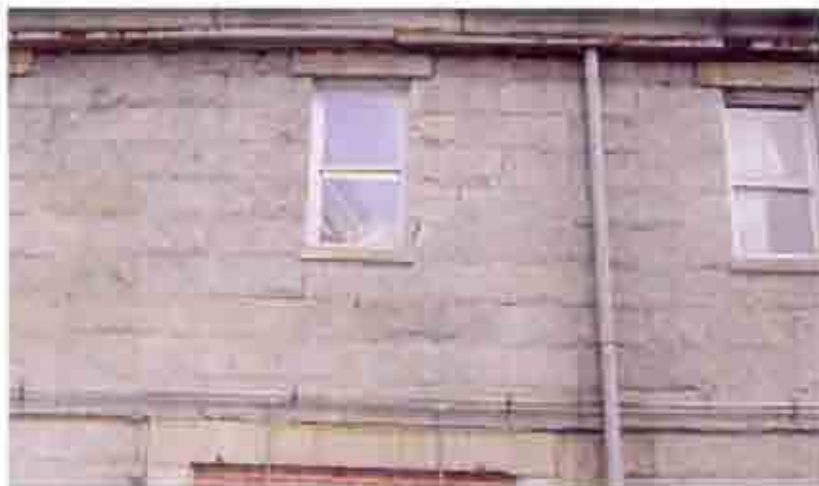
Fig. 27. West elevation, third door opening from the north. Note step cracking from the left of the door to the lintel of the right window. Door lintel is out of level.
