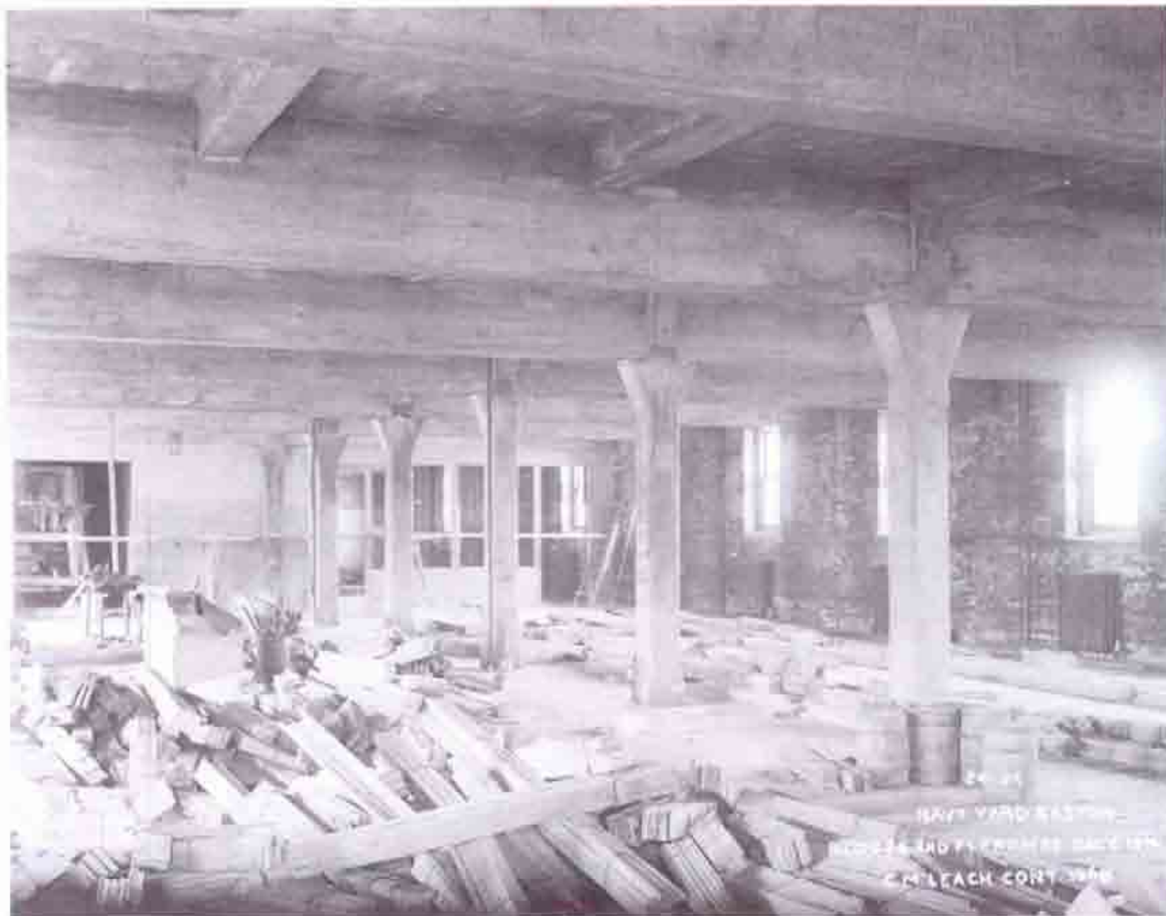
Fig. B-29 Photo "24-27 NAVY YARD BOSTON BLDG 24 2ND FL FROM S.E. DEC. 3, 1914 C. M. LEACH CONT 1968". Second floor interior, looking north. Concrete poured for floors and column casings. Bundled wood (probably flooring material) stockpiled on floor.
