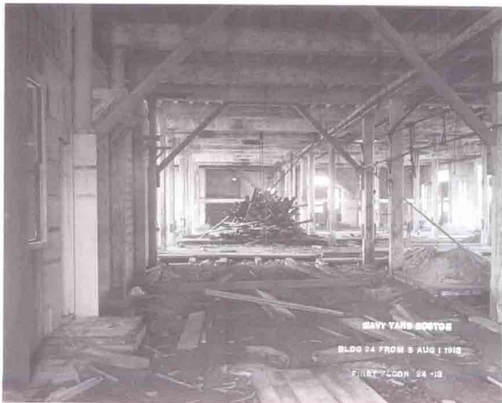
B14 Fig. B-14 Photo "NAVY YARD BOSTON BLDG 24 FROM 5 AUG 1 1913 FIRST FLOOR 24-13". Interior showing progress of demolition.
