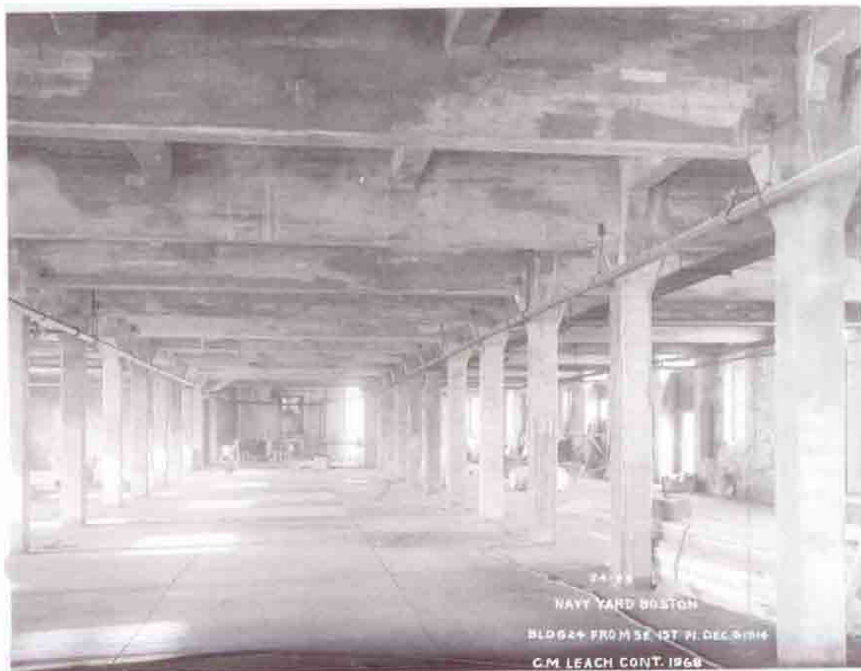
Fig. B-28 Photo "24-26 NAVY YARD BOSTON BLDG 24 FROM SE. 1ST FL. DEC. 3 1914 C. M. LEACH CONT. 1968". First floor interior, looking north. Concrete poured for floors and column casings. Windows installed. Still under construction.
