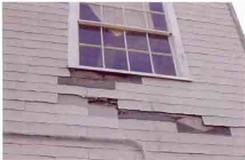
Fig. 20 Detail of asbestos shingle siding and window condition
