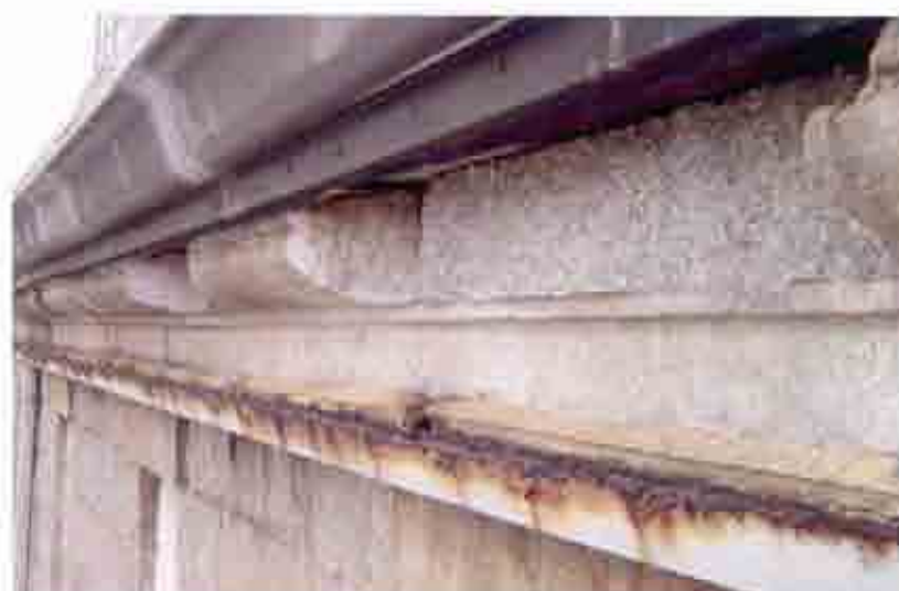
Fig. 8 West elevation cornice stone with spalled stone, rusted gutter fasteners, and rusted Z channel.
