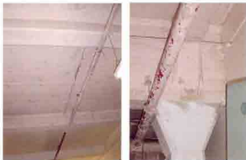
Fig. 34& 35 Typical construction shrinkage crack in concrete slabs (left), and vertical crack at beam-to-column intersection (right).
