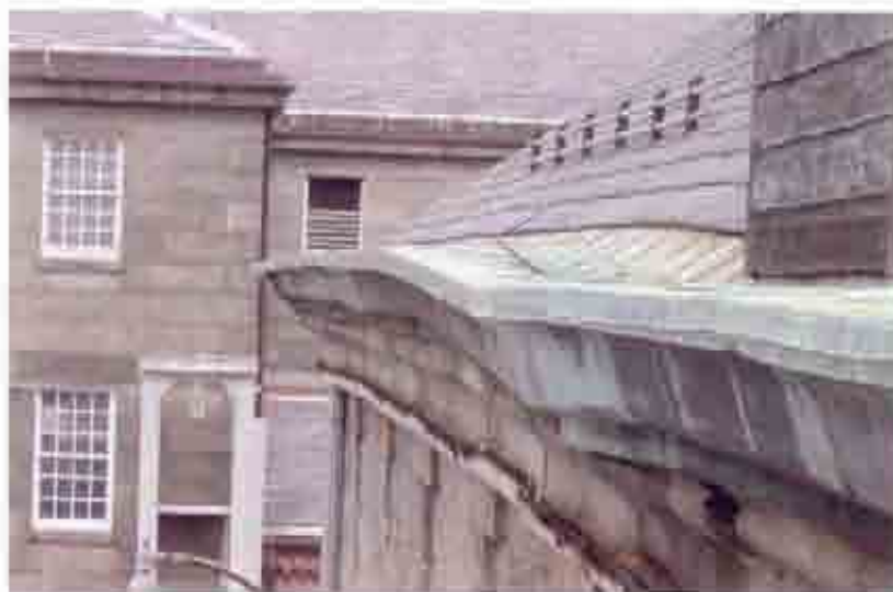
Fig. 30 West elevation cornice, looking north. Note dip in gutter level and rusted Z channel.
