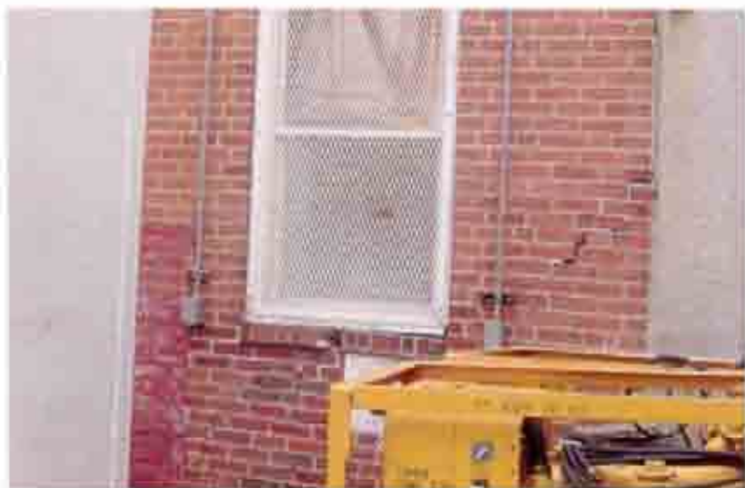
Fig. 28 West elevation, step crack detail. Continuation of crack into brick infill panel.
