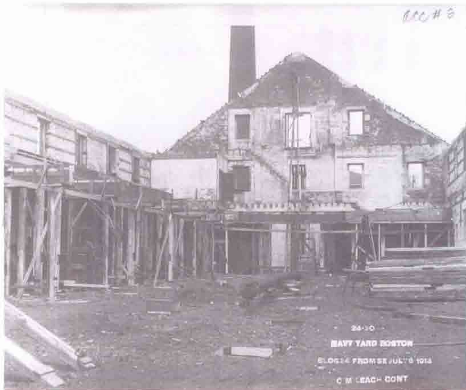
Fig. B-21 Photo "24-20 NAVY YARD BOSTON BLDG 24 FROM SE JULY 6 1914 C M LEACH CONT". First floor interior, looking north. Formwork started for poured concrete floor structure.
