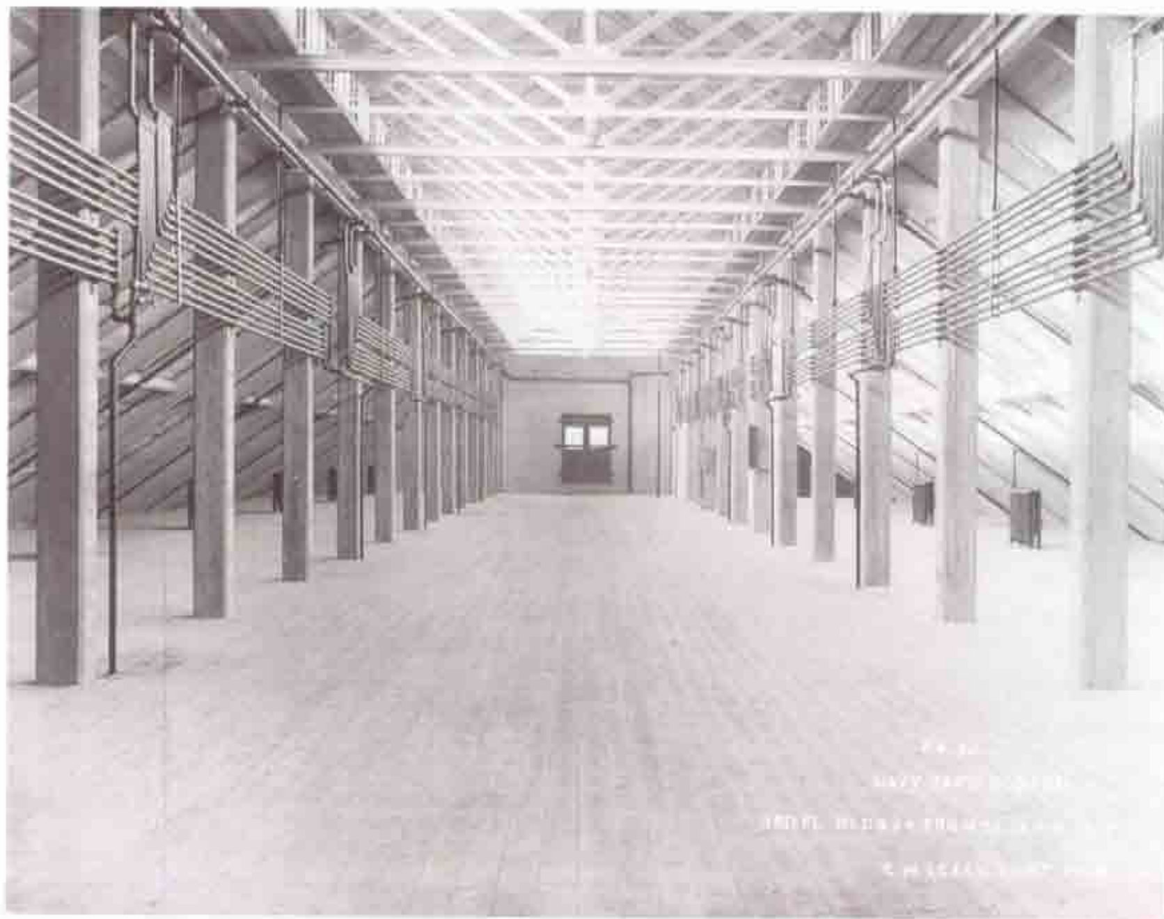
Fig. B-31 Photo "24-32 NAVY YARD BOSTON 3rd FL BLDG 24 FROM S.E. JAN 4 1915 C.M LEACH CONT 1968". Third floor interior, looking north. Work complete, radiators in place along perimeter eaves, piping along columns.
