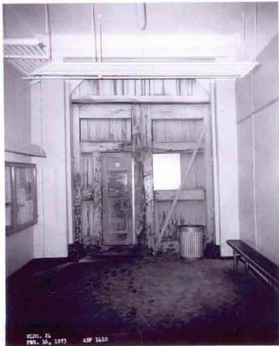
BS4 Fig. B-54 Photo "BLDG. 24 FEB. 16, 1973 ASF 1410". 1973 photo showing cracked lintel over door.
