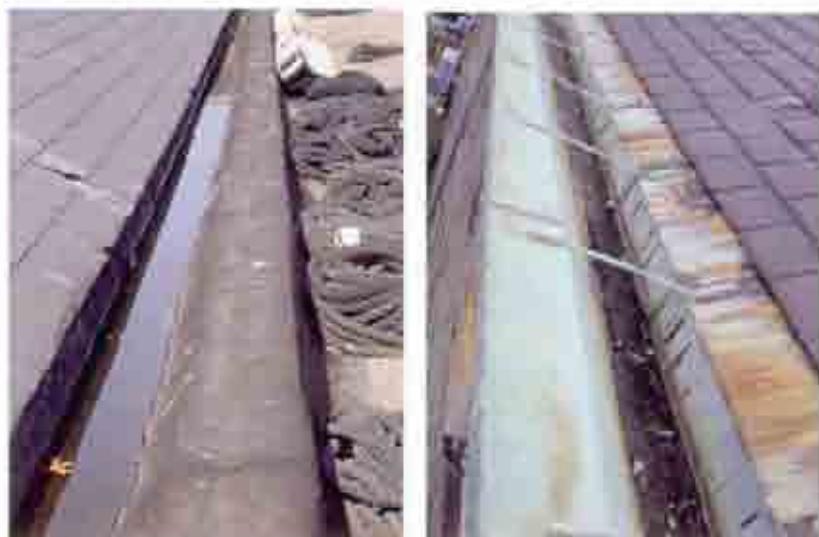
Fig. 12 & 13 East roof slope (left) with original copper gutter coated to meet fast roof of addition. Copper gutter of west roof slope (right) shows streaking, indicating advanced deterioration of material.
