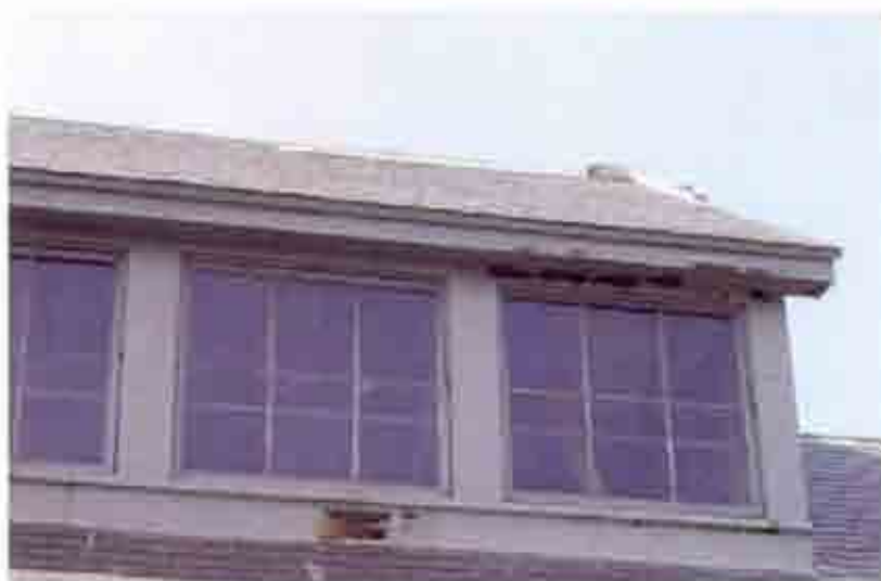
Fig. 17 Monitor. Detail of wood windows and metal trim. Note rusting of galvanized metal and loss of paint on wood and metal.
