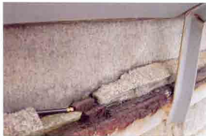
Fig. 9 West elevation cornice stone. Note mortar filler in gap created at Z channel.
