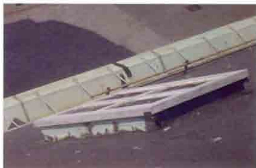
Fig. 14 Many of the wood framed skylights are actively leaking. Note the loss of paint and patched metal flashing.
