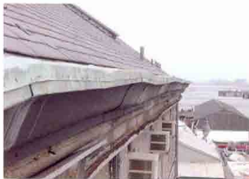
Fig. 31 West elevation cornice, looking south. Note dip in cornice stone and rusted Z channel.
