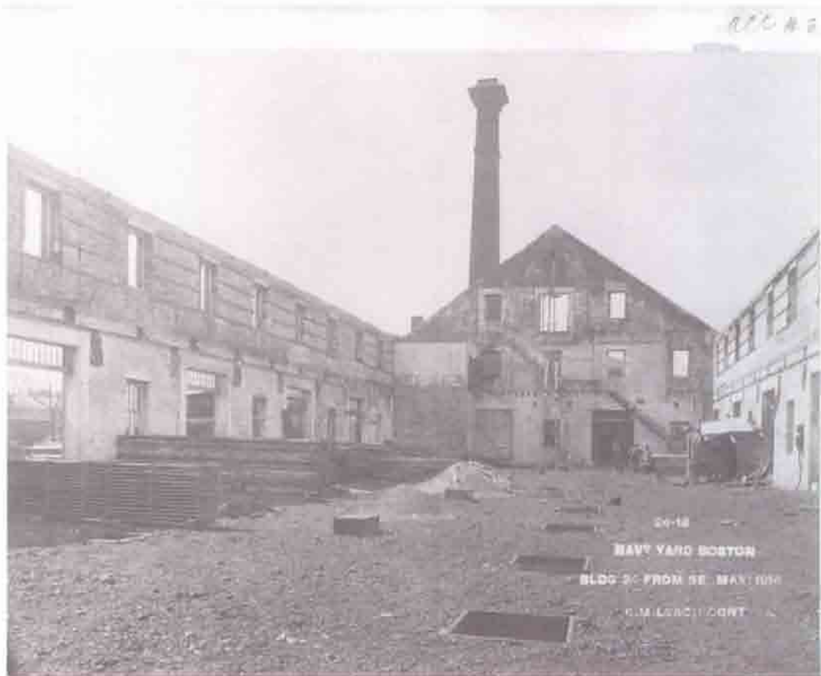
Fig. B-19 Photo "24-18 NAVY YARD BOSTON BLDG 24 FROM SE MAY 1 1914 C. M. LEACH CONT". First floor interior, looking north. Pockets formed for column footings. Material stocked for reconstruction.
