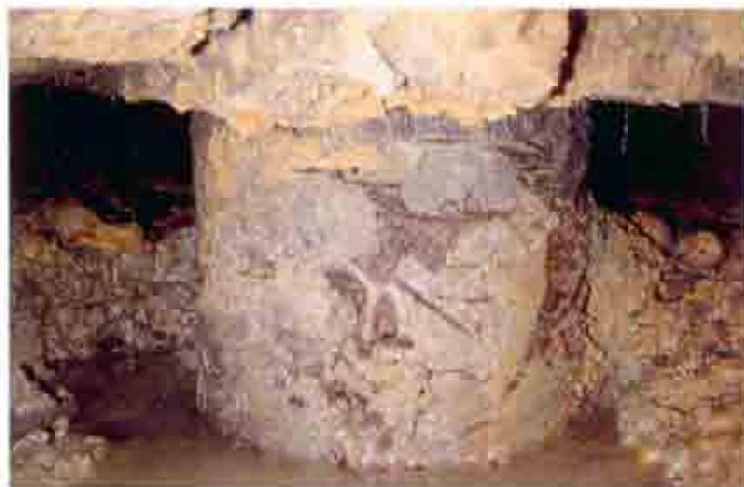
Fig. 38 Groundwater was observed entering Test Pit No. 2 at a depth of about five and a half feet.
