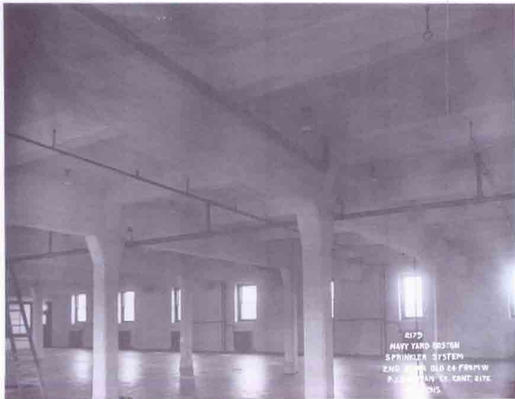
Fig. B-34 Photo "2179 NAVY YARD BOSTON SPRINKLER SYSTEM 2ND FLOOR BLD 24 FROM W.P. SULLIVAN CO. CONT. 2173 (?) OCT 1, 1915". Second floor interior, looking east. Sprinkler system in place.
