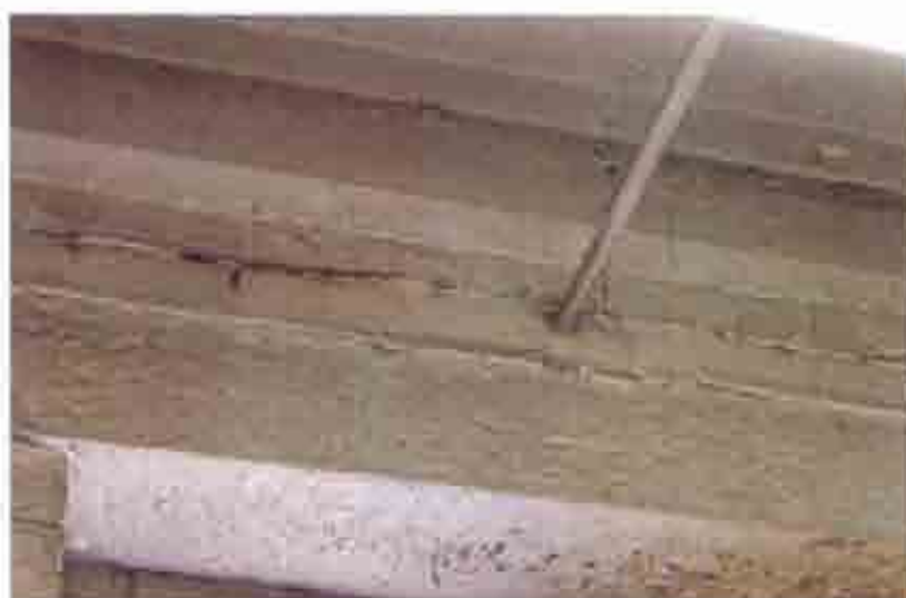
Fig. 33. Typical condition where Z channel tie rods pass through exterior wall.
