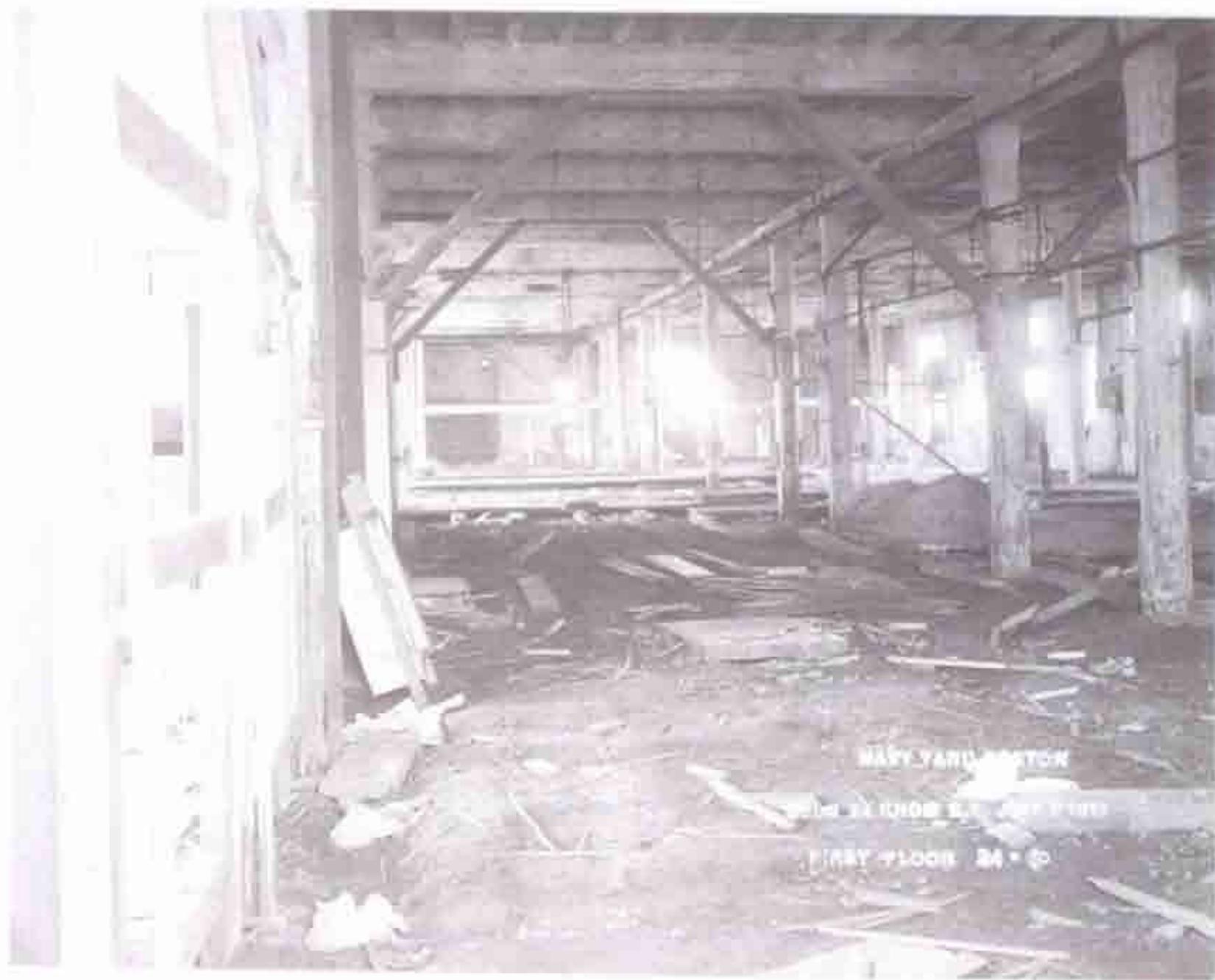
Fig. B-11 Photo "NAVY YARD BOSTON BLDG 24 FROM S.E. JULY 2 1913 FIRST FLOOR 24-10". Interior photo of original wood columns and beams.
