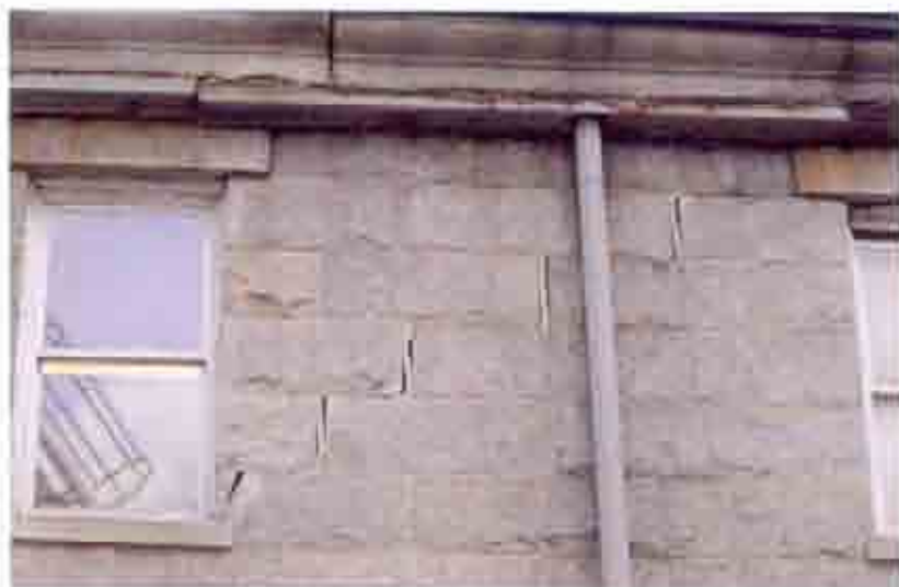
Fig. 7 Step cracks have formed along some mortar joints due to structural movement of the building.
