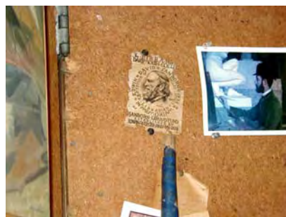
Silverfish Damage on Wall
