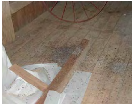
Bat Droppings under Beam
