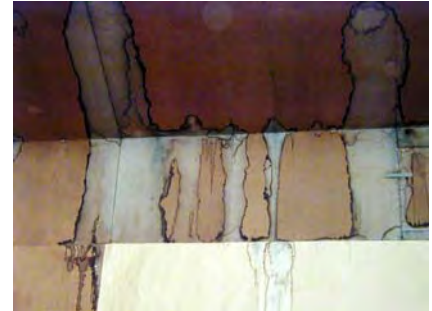
Old Water Damage Stain
