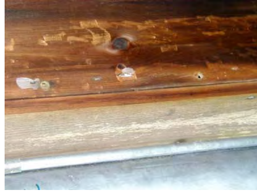
Carpenter Bee Damage
