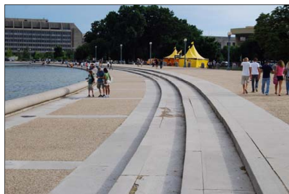
Grade level changes at Union Square and deteriorated paving make access difficult for visitors in wheelchairs.
