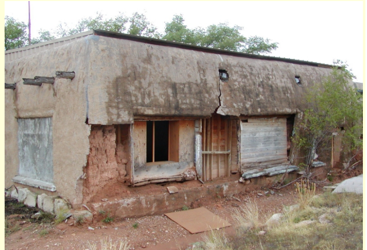
Deteriorated north wall of bath house, before repair.
