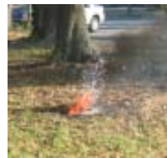
Fire pit that used to be Electrical Junction Box
