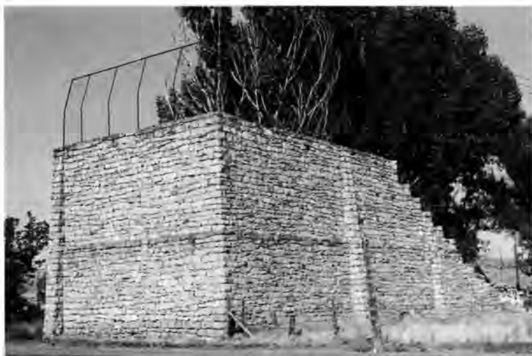
A National Register property associated with Basque culture, the Pelota Fronton in Jordan Valley, Oregon, was constructed in 1915 and used up until the 1930s. The fronton, or court, was the gathering place for Basque immigrants to play the traditional handball game of pelota. Courtesy Oregon State Historic Preservation Office.
