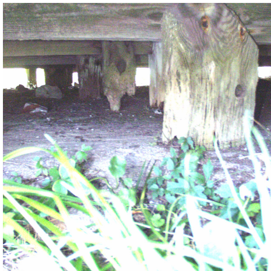
Figure 2 View of rotted wooden piers that formerly supported floor joists at mid-span. (NPS-SERO-CRS, 2002)
