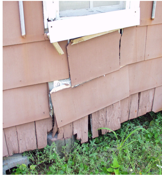
Figure 6 View of damaged siding on northeast side of house, the result of major sill damage in this location. Original board siding is exposed across bottom of wall. (NPS-SERO-CRS, 2002)
