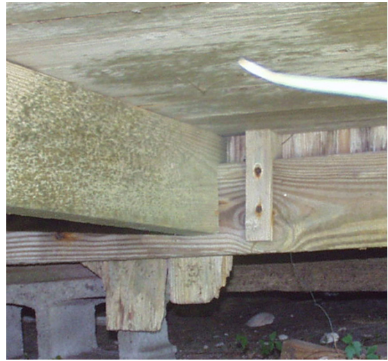
Figure 3 View of front sill of house and typical joist and stud connections. (NPS-SERO-CRS, 2002)
