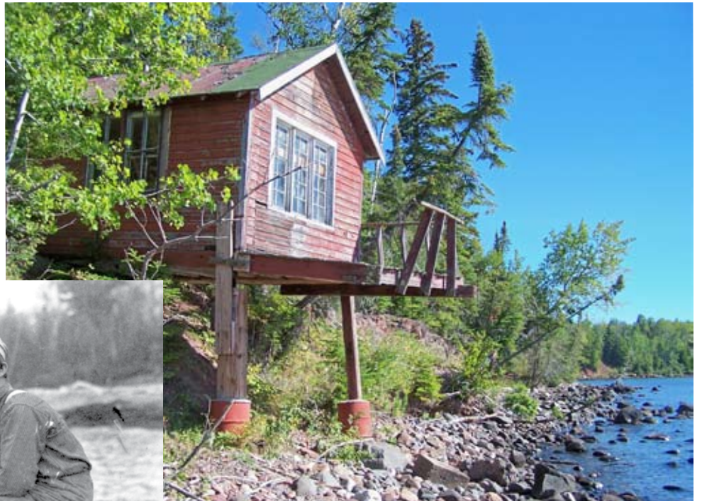
The Boar's Nest, one of the Hansens' guest cottages, needs to be moved back from its precarious perch on the edge of the bank bordering East Bay,
