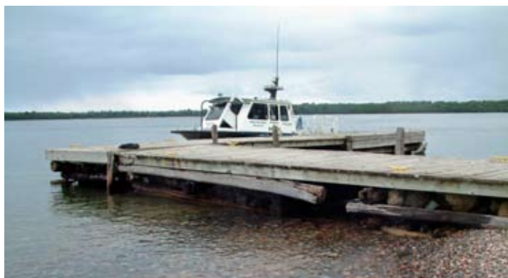
Top: Repairs to the Fresnel lens and lantern room windows in the Devils Island tower are scheduled for this summer.
