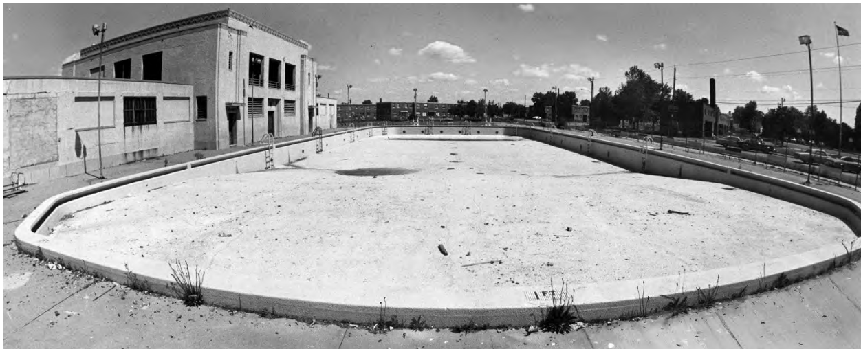
Figure 5: Abandoned swimming pool that was a part of a recreational center in Camden, New Jersey, June 20, 1978. Photographed by Joe Del Palazzo. Courtesy of the George D. McDowell Philadelphia Evening Bulletin Collection, Temple University Special Collections Research Center
