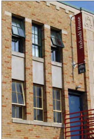
[21] The windows on the lower floor, which were too deteriorated to repair, were replaced with new steel windows matching the upper-floor historic windows that were retained.
