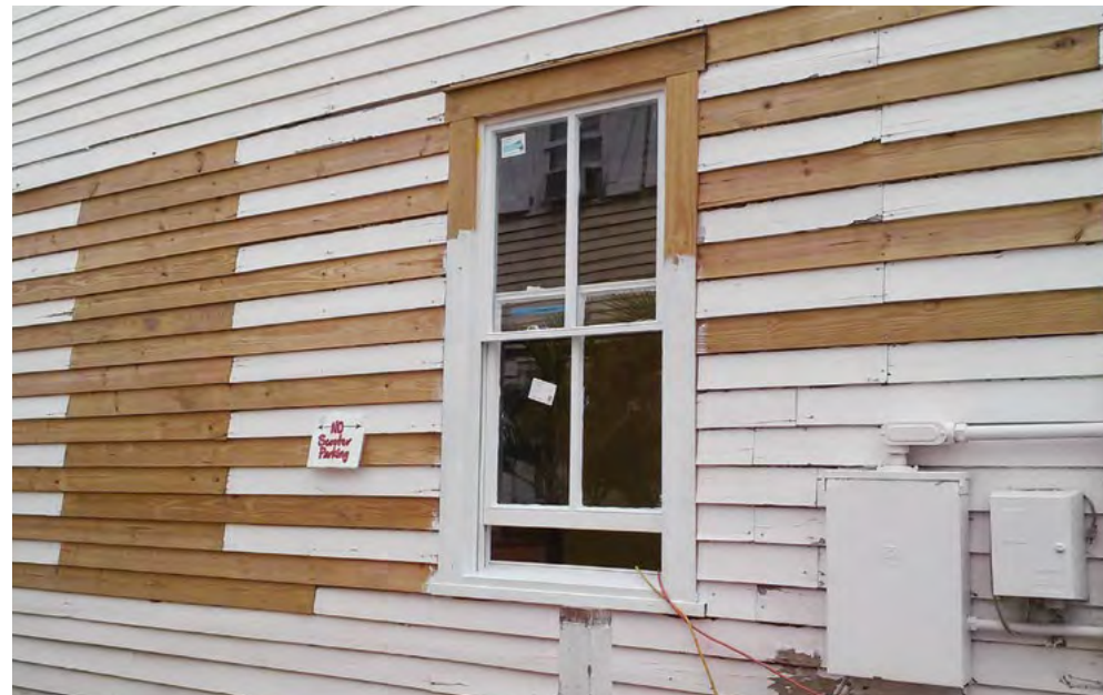
[8] Rotted clapboards have been replaced selectively with new wood siding to match the originals.
