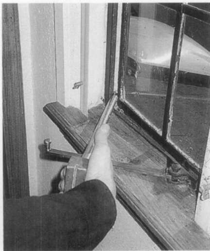
Figure 6. Pull bars were used to realign the sash from the inside. These custom made tools were especially useful on single sash units where the worker was unable to reach through an adjacent opening to apply pressure from the outside.
