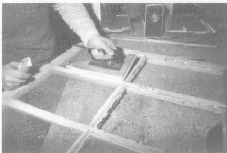
Figure 3. Electric deglazing irons were used to remove hardened putty so glass could be removed and the sash frames repaired. Photo: Christopher Closs
