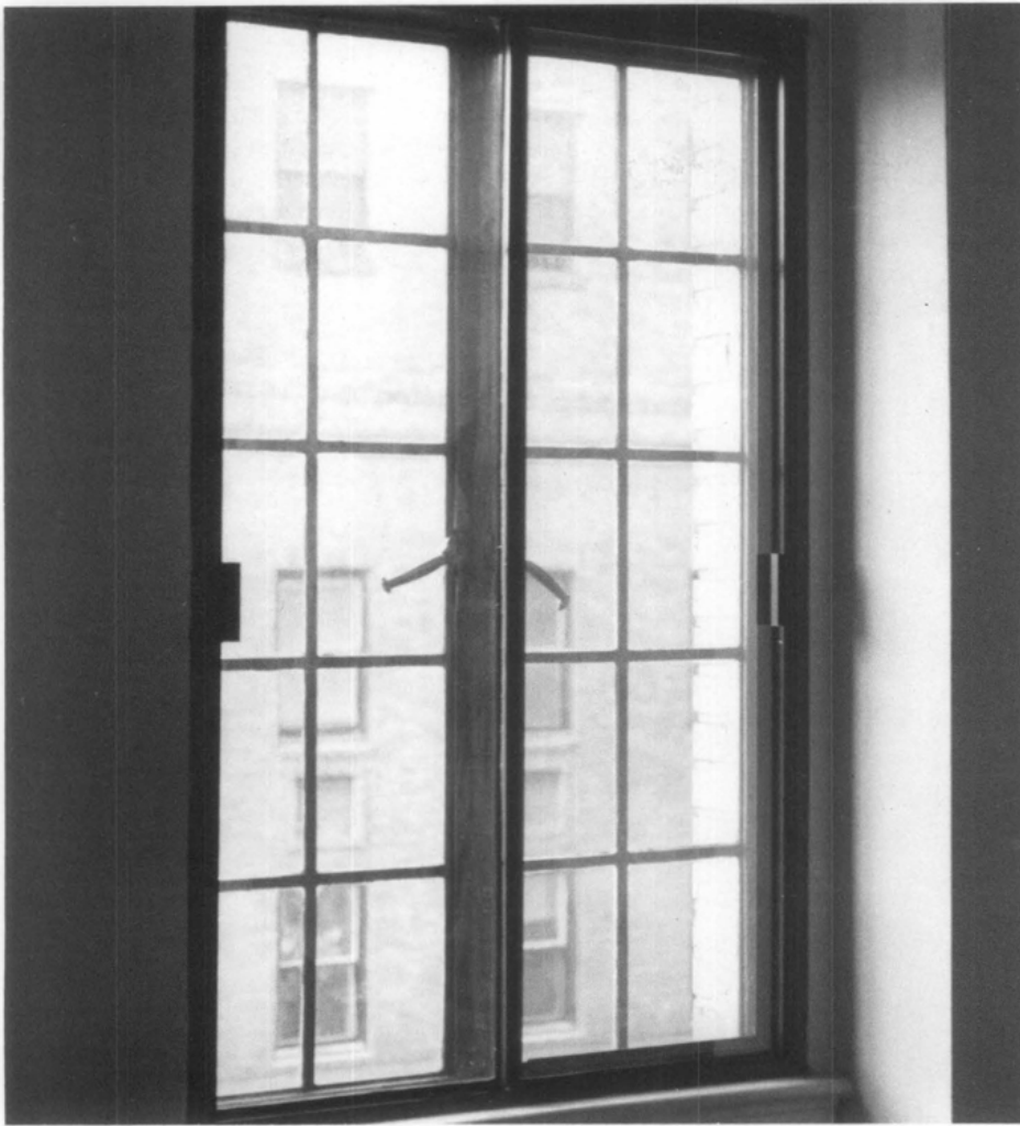
Figure 2. A horizontally sliding storm window unit was installed on the inside of the casement windows for improved energy performance. Photo: Christina Henry.
