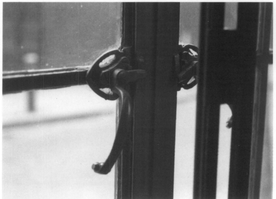
Figure 4. The hardware was cleaned and oiled as part of the maintenance and repair work undertaken on the steel casements. Photo: Charles Fisher.
