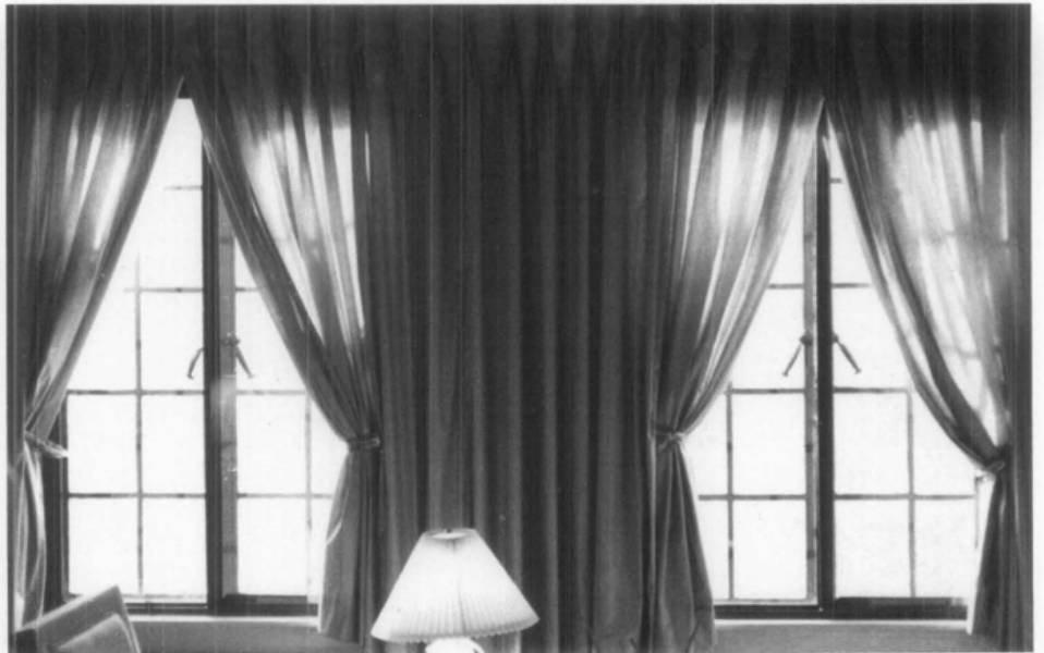
Figure 8. The storm units are neatly set within the opening and aesthetically are not disruptive. Photo: Charles Fisher.
