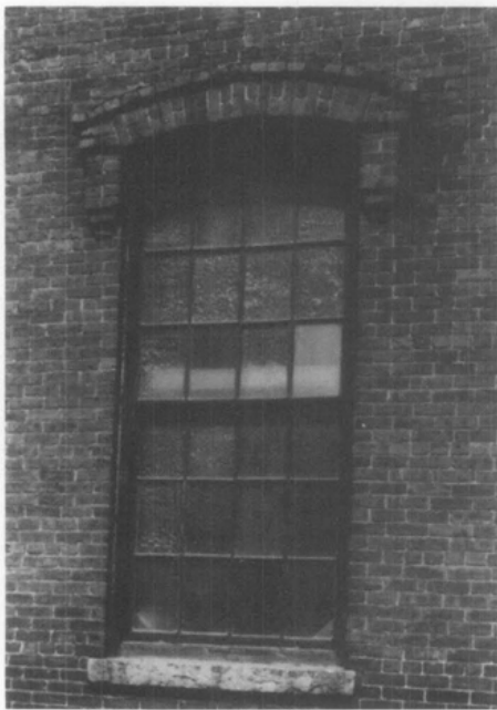
Figure 1. The original wooden double-hung windows consisted of 12 lights in both the upper and lower sash. Photo: Charles Parrott
