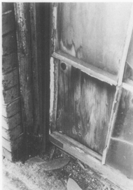
Figure 2. The condition of the windows varied considerably. Shown here is a typical case where the frame, sill and sash were beyond repair. Photo: Charles Fisher
