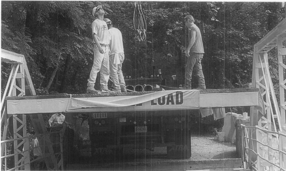
Figure 10. When the deck arrived at the site, the trailer was backed onto the bridge approach and crane cables secured to the deck. Although the road beyond that side of the bridge is a dead end, the truck driver was able to maneuver across a vacant site to get the deck on the opposite side of the creek.
