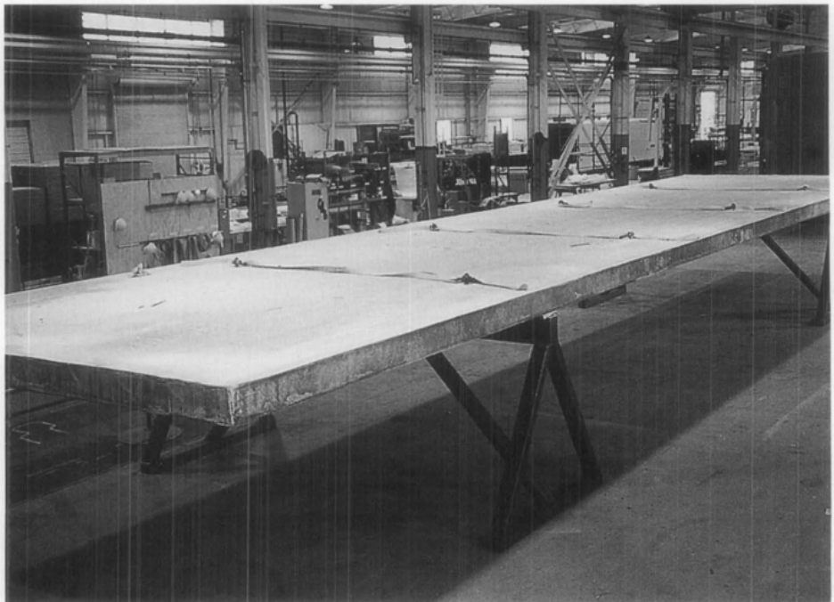
Figure 7. After the panel had set into a solid mass, workers removed it from the mold and sanded and finished all surfaces. The last steps included painting the deck and installing the oak plank wearing surface. Photo: Hayati Catbas, Hardcore Composites.
