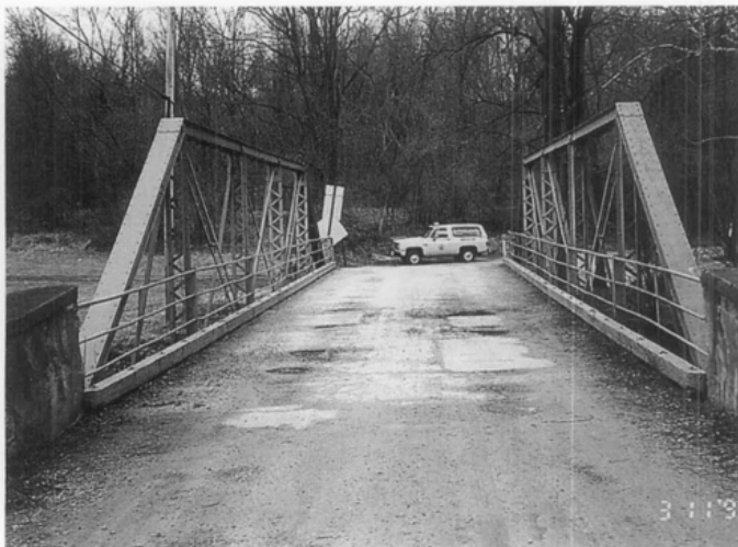
Figure 2. Before rehabilitation, Wilson's Bridge had an asphalt wearing surface that was delaminating from the deck below. Extensive cracks and numerous potholes were also present.
