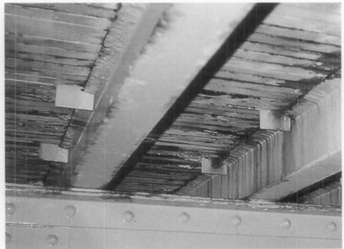
Figure 3. A view of the underside of Wilson's Bridge before rehabilitation. The timber nail laminated deck sat on steel "I-beam" stringers which, in turn, were supported by wrought iron floor beams. Failure of the wearing surface had allowed water to penetrate the laminated deck planks causing further deterioration to both the deck and the stringers below.
