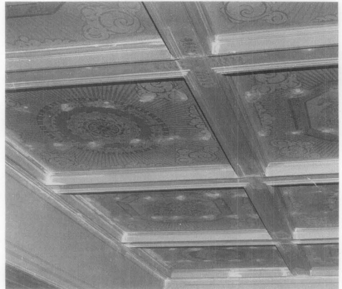
Figure 14. Holes left by insertion of toggle bolts used in the structural strengthening of this ceiling can be seen in the decorative plaster work. Without great expense, a skilled painter can now clean and touch up the damaged areas. This type of targeted repair work can benefit both public and private buildings. Photo: National Park Service files.
