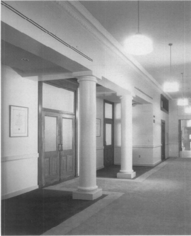
b. Central air conditioning was installed in the corridors of this circa 1900 school building by adding an air handler over the entrance from a vestibule. The custom-designed slot registers provide linear diffusers without detracting from the architecture of the space. Photo: Lautman Photography courtesy of Notter Finegold + Alexander Inc.
