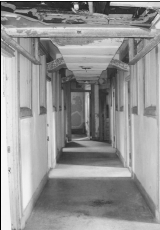
Above: The dropped ceiling has been partially removed, revealing the old ductwork running through the center of the hallway and branching into each office. The ceiling had been lowered from its historic height of 10 feet to just 7 feet.
