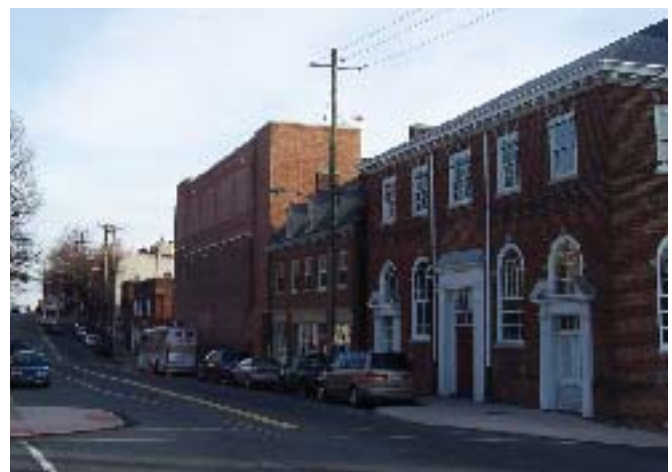
The new fly loft redesigned to meet the Standards is shown here after rehabilitation.
