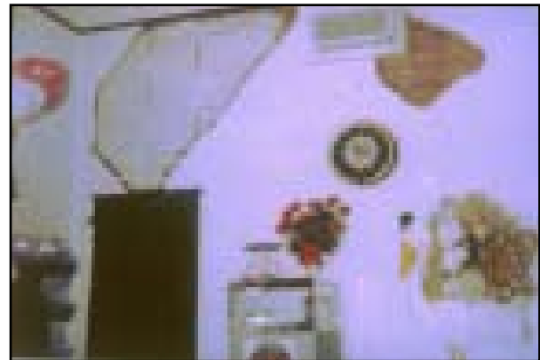
During the rehabilitation, a tenant left an area of the wood lath exposed when repairing the plaster walls in an office space. This treatment was not compatible with the historic character of this traditionally finished space, and the plaster had to be repaired before the project could meet the Standards.
