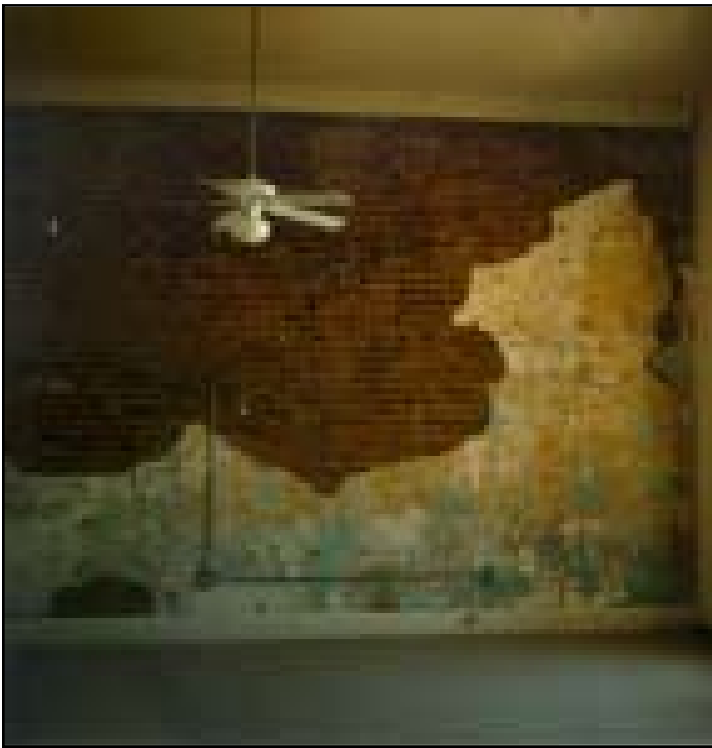
Keeping deteriorated plaster fragments as found without repairing the plaster finish is not an appropriate rehabilitation treatment for most historic building interiors.
