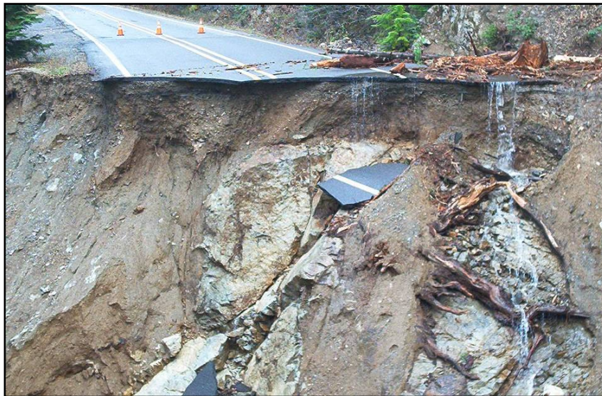
State Route 123 was heavily damaged during the flood.
