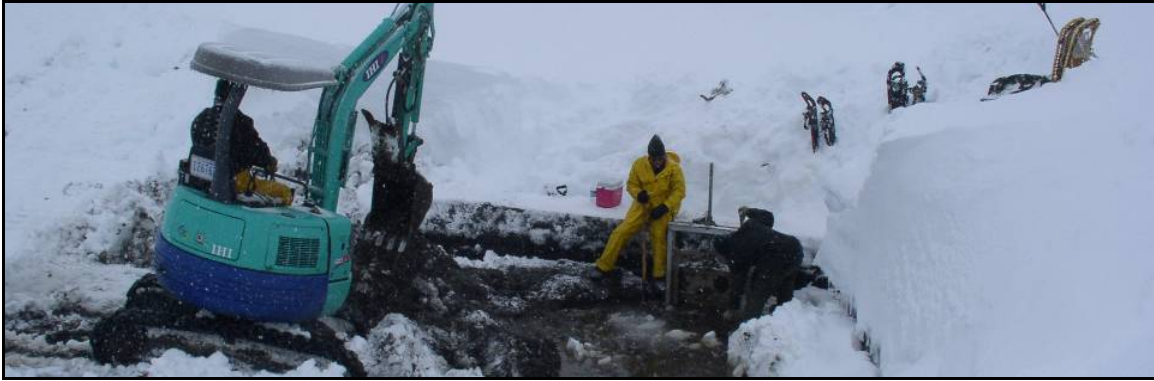
Power, sewer and water utilities were restored, despite 10 feet of snow on the ground at Paradise.
