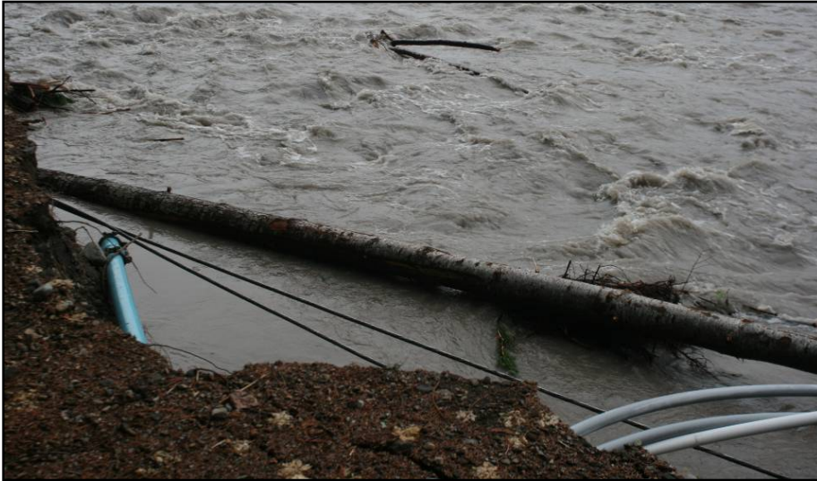
The park's buried power line was destroyed for a length of 1200 feet at Sunshine Point, shorted out at Kautz Creek and exposed by erosion in two other places. The overhead line to the water treatment plant at Longmire was also broken.
