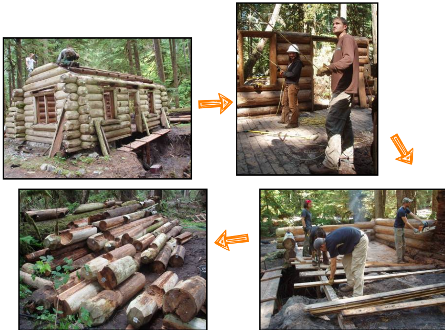
The historic Ipsut Creek Patrol Cabin, undermined by flood waters, was deconstructed in August and transported to Tahoma Woods for restoration.
