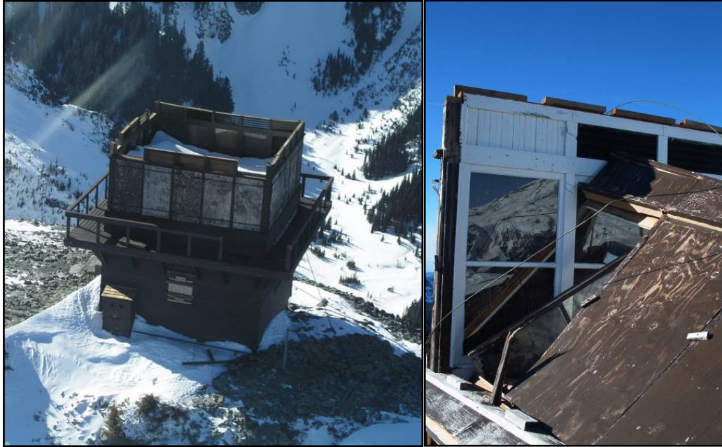
High wind tore the roofs from the Fremont and Gobbler's Knob Fire Lookouts.
