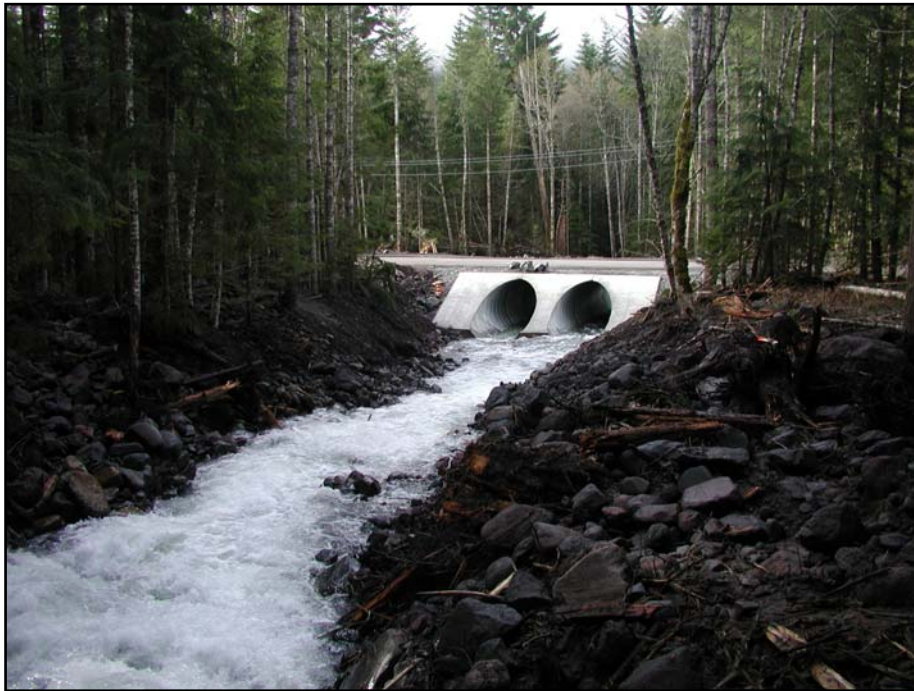
Two 12- foot culverts accommodate the new Kautz Creek channel at Nisqually Road.
