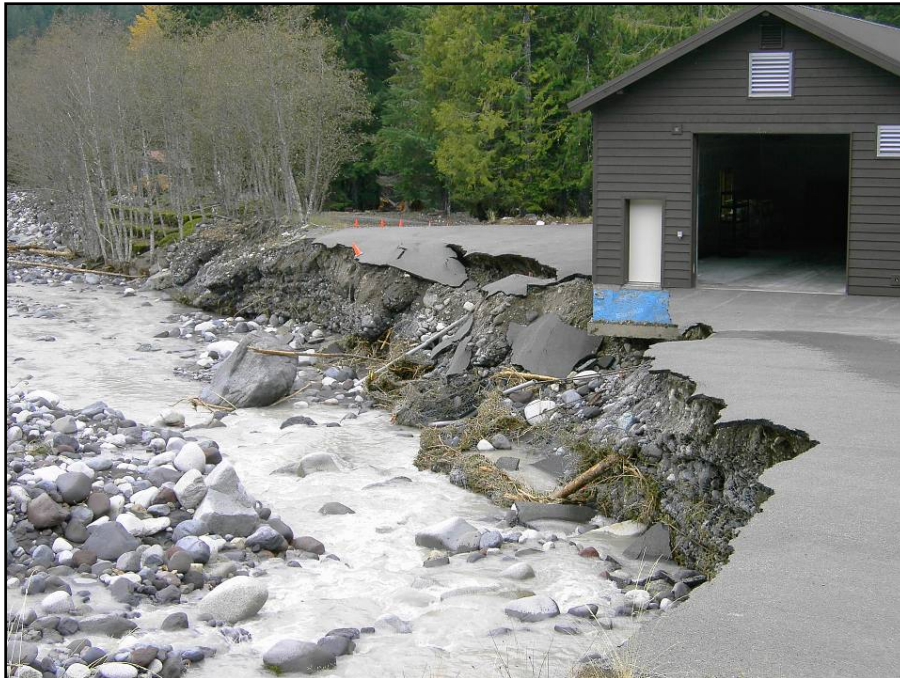
The Emergency Operations Center at Longmire was especially vulnerable. Sixty feet of levee and river bank eroded away during the storm, leaving one corner of the building hanging over empty space.
