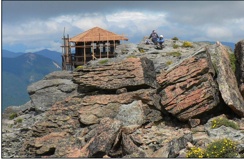
Mount Fremont and Gobbler’s Knob Fire Lookouts now have roofs and interior restoration will continue into 2008.
