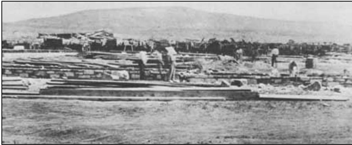
Construction scene at the third Fort Union and depot, date and particular building unknown. U.S. Signal Corps Photo No. 87995, courtesy National Archives.
