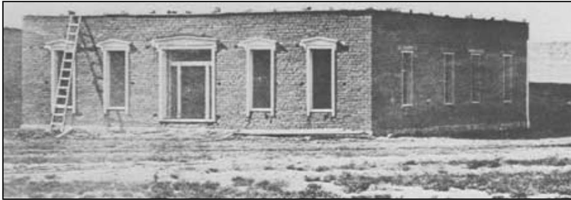
Officer's quarters under construction at third Fort Union, U.S. Signal Corps Photo No. 88013, courtesy National Archives.
