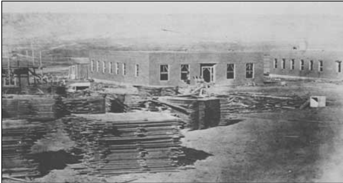
Officers' quarters under construction at third Fort Union. The site of the first fort is barely visible in left background at base of bluffs. U.S. Signal Corps Photo No. 87997, courtesy National Archives.
