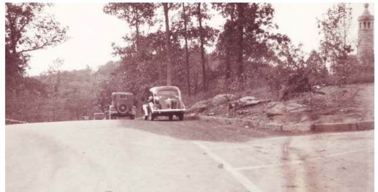
Figure 2.40. New Sykes Avenue parking lot, cut into the east slope of Little Round Top, ca. 1936 (GNMP General Historic Photographic Prints GETT 41135 #SF-22R-068).
