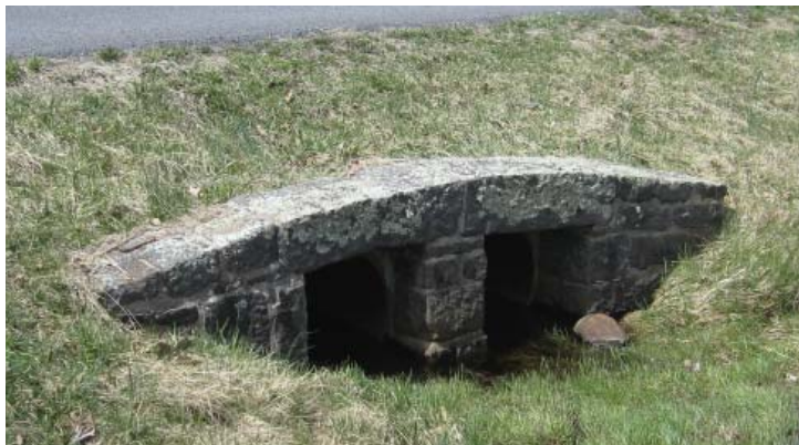
Figure 3.89. NPS Era round-topped stone culvert, constructed by the Civilian Conservation Corps (Photo by RHI, 2011).
