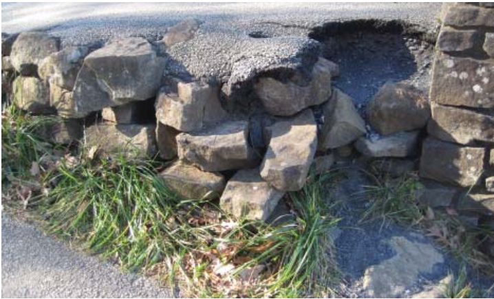
Figure 3.19. Asphalt paths show significant erosion at the edges. These paths line the summit of Little Round Top (Photo by RHI, 2010).
