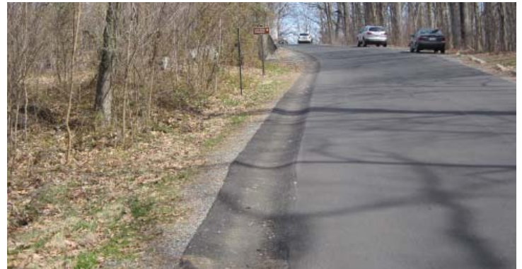
Figure 3.91. Asphalt gutter on the west side of Sykes Avenue (Photo by RHI, 2011).
