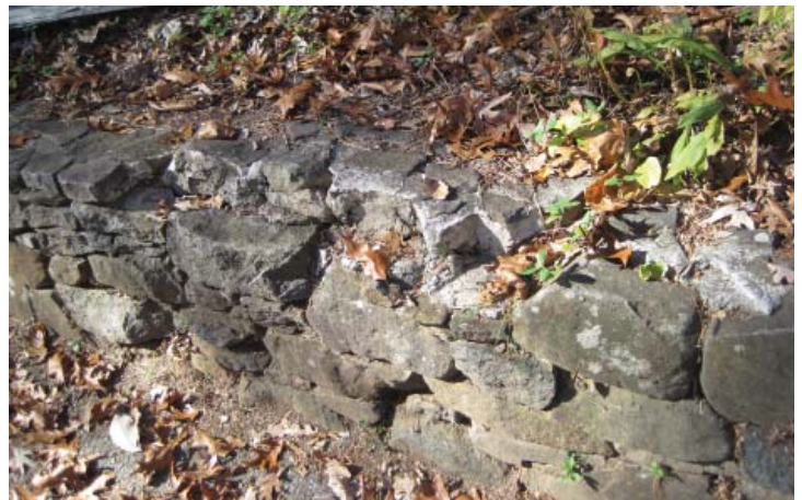
Figure 3.75. Damage to the cap of the stone and mortar retaining wall at the Sykes Avenue parking area (Photo by RHI, 2010).
