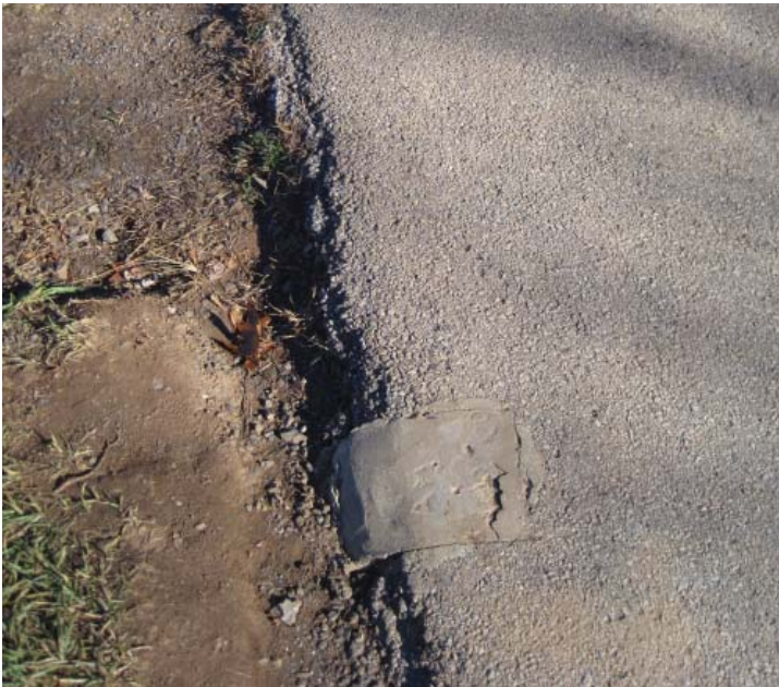
Figure 3.78. Remnant of the post-and-chain system installed to keep visitors on the asphalt paths at the summit of Little Round Top (Photo by RHI, 2010).
