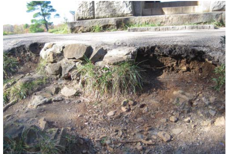
Figure 5.04. An example of degradation to the pathway system at the summit of Little Round Top. Deteriorating conditions such as this cause damage to the surrounding unimproved terrain through increased erosion and compaction from visitors stepping off the path (Photo by RHI, 2010).
