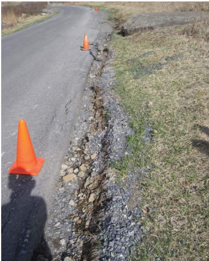
Figure 3.93. Undercutting of the roadbed along the north side of Warren Avenue has caused a partial failure of the roadway (Photo by RHI, 2011).
