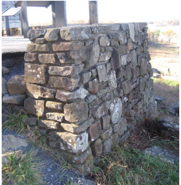
Figure 3.74. Stone and mortar retaining wall at the summit of Little Round Top (Photo by RHI, 2010).
